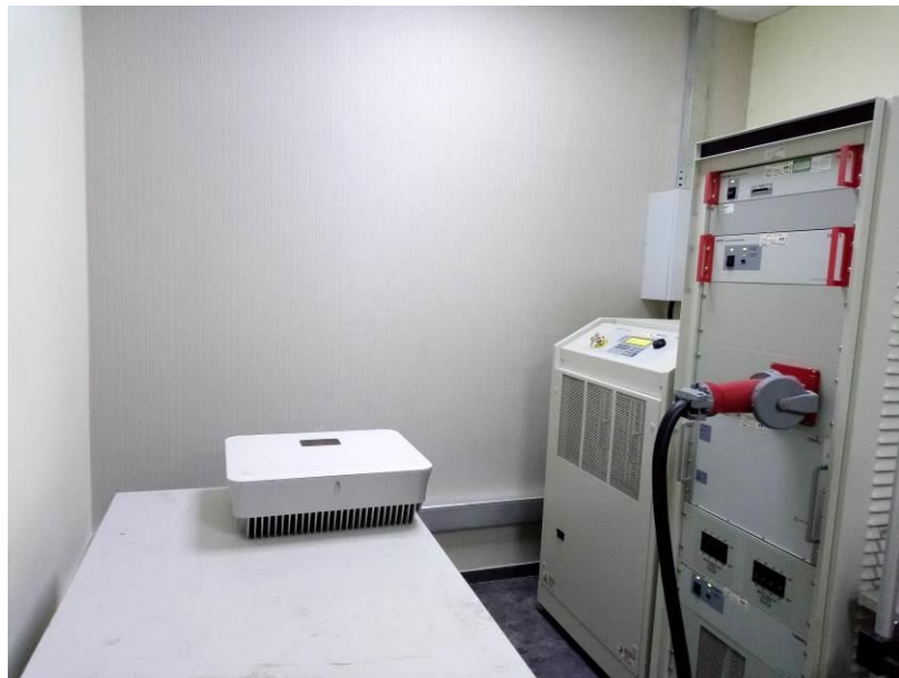
Figure 7 Voltage fluctuations and flicker test setup
