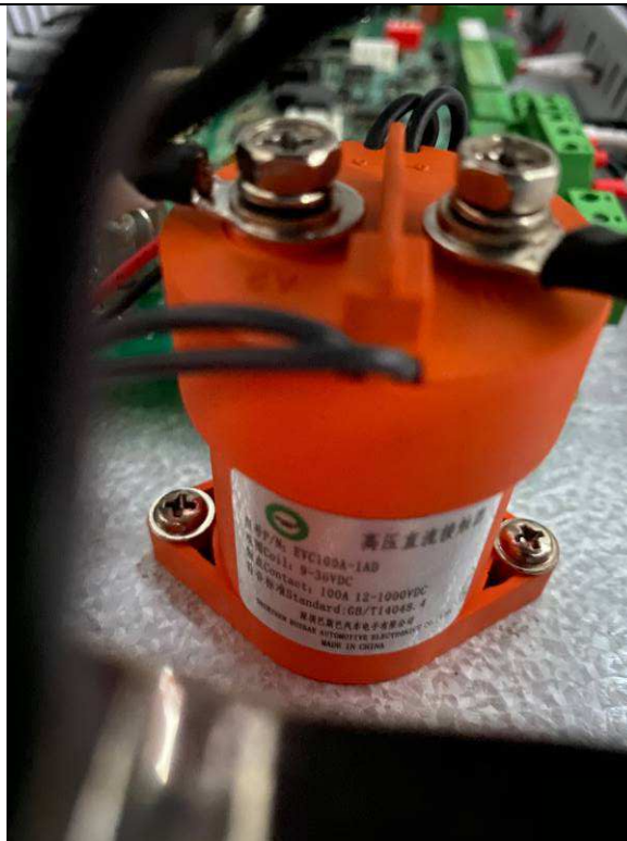
Figure 14 DC contactor (pre-charge)
