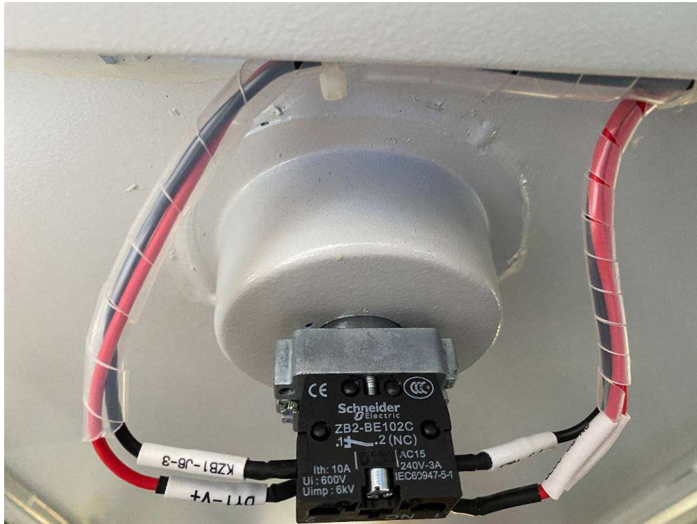
Figure 21 emergency stop switch
