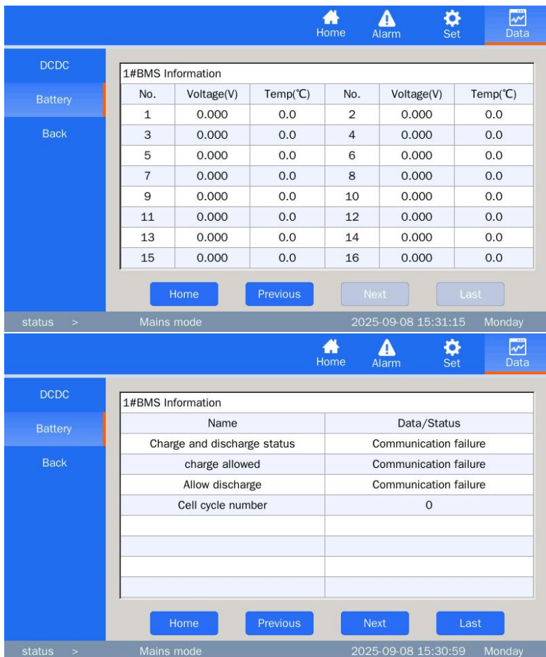
Figure 3-36 Battery Status Interface
